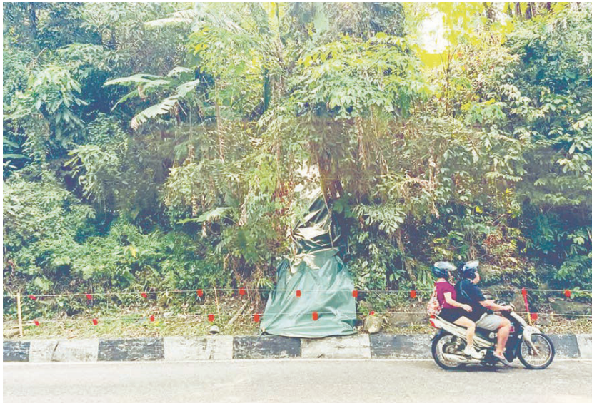
Safety sheets have since been placed at the site to prevent further soil movement. - PIC FROM ZAIRIL KHIR JOHARI FACEBOOK PAGE
