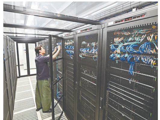
CCB's property division generated 88% of revenue, 75% from NCIP data centre land sales. - AFPPIX
