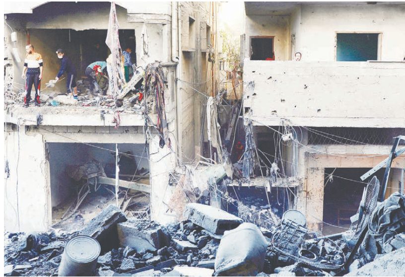
Palestinians inspect the damage at the site of a strike at the Nuseirat refugee camp in central Gaza Strip. – REUTERS/PC
