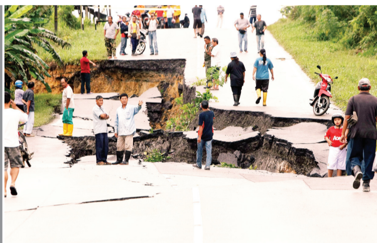
ON CRACKING LAND ... A road in Serian, Sarawak had massive cracks after continuous heavy rains.
