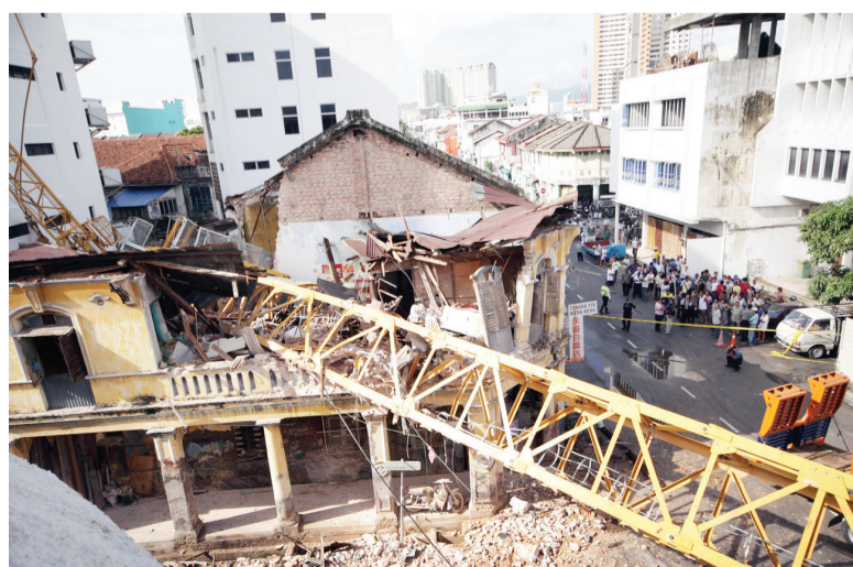
CRANE CRASH ... A seven-storey crane tower crashed on a pre-war shophouse in George Town, killing one and injuring three others. The tower had toppled from a nearby construction site onto the house, burying 65-year-old Liang Yit Kwang under the debris in early October.
