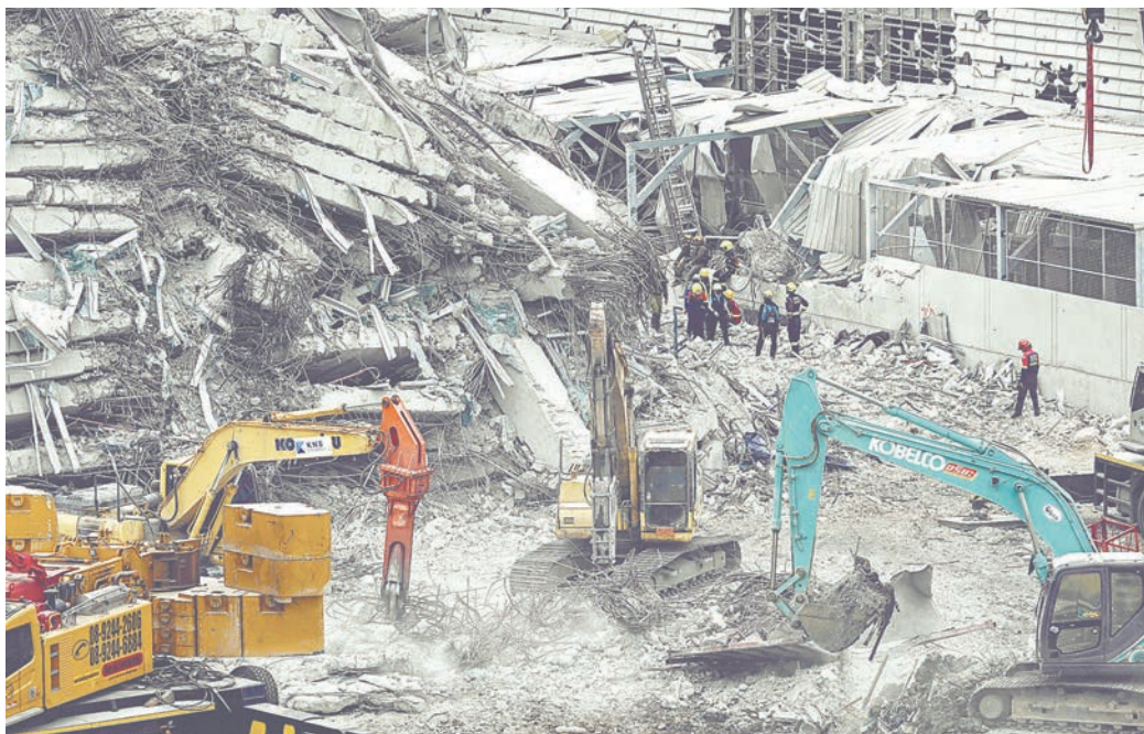
Heavy machinery is used to clear the debris at the site of the collapsed building collapse in Bangkok yesterday. — AFP/PPIC
