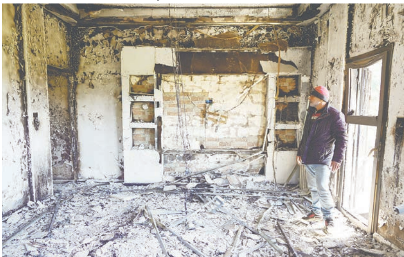
A resident of Jableh, Abu Ali al-Khair, inspecting his damaged house on Wednesday. – REUTERSPIC
